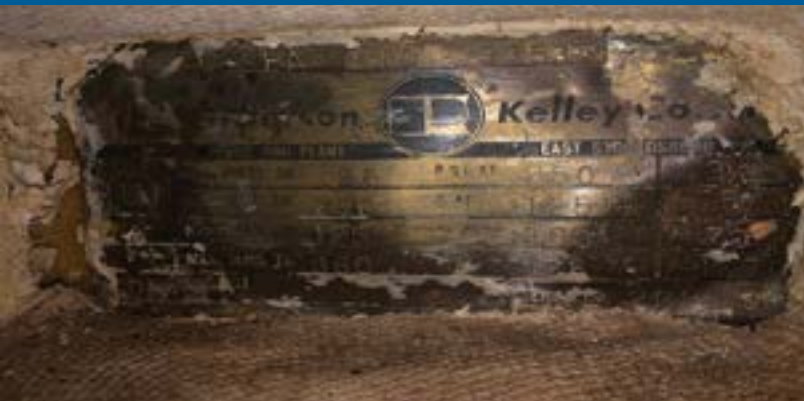
Patterson-Kelley Original 1970 Water Heat Tag (Pictured Above)
